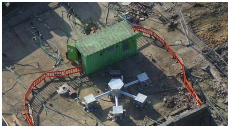
Fig. 2 Container-based modular system with the RF generator and the matching network in combination with an arrangement for soil vapour extraction
