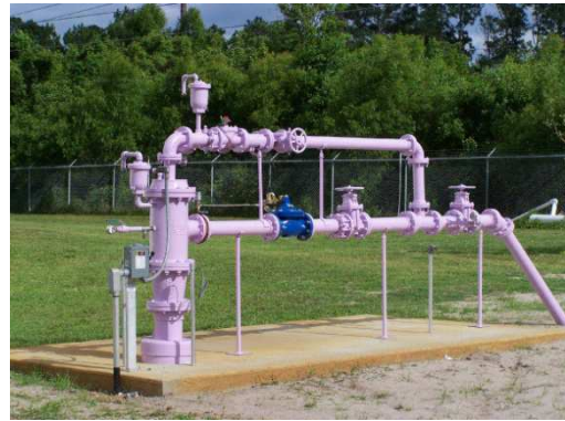
Figure 1 - Destin ASR system wellhead
